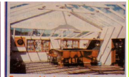
Damaged by hurricane Luis
